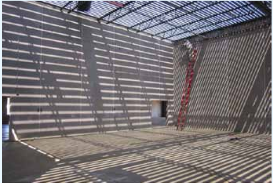
Construction crews are busily erecting a new 37,000-square-foot permanent school building for Imagine Andrews.
